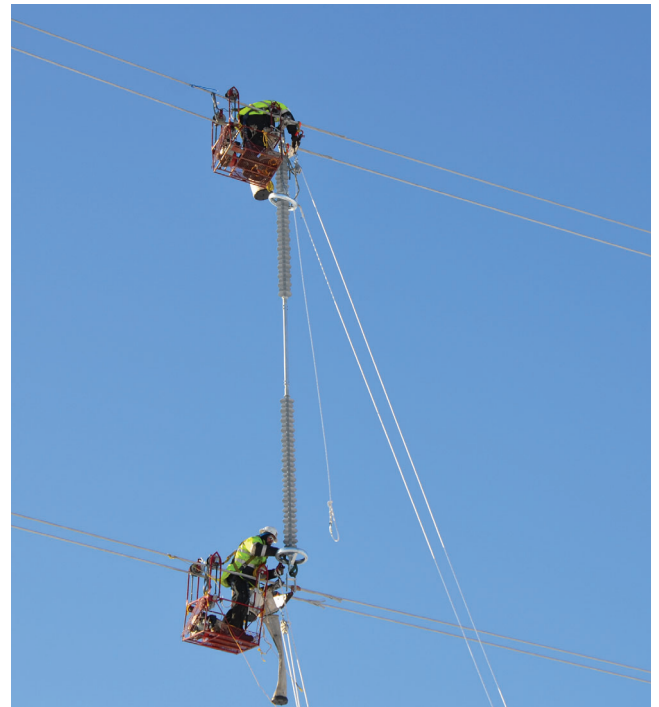
Workers use buggies attached to conductor to install the interphase spacers. The devices weigh nearly 200 pounds and 25 feet long.
