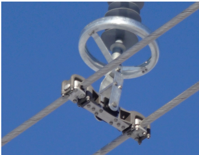
The spacer is attached to the conductor on both ends
