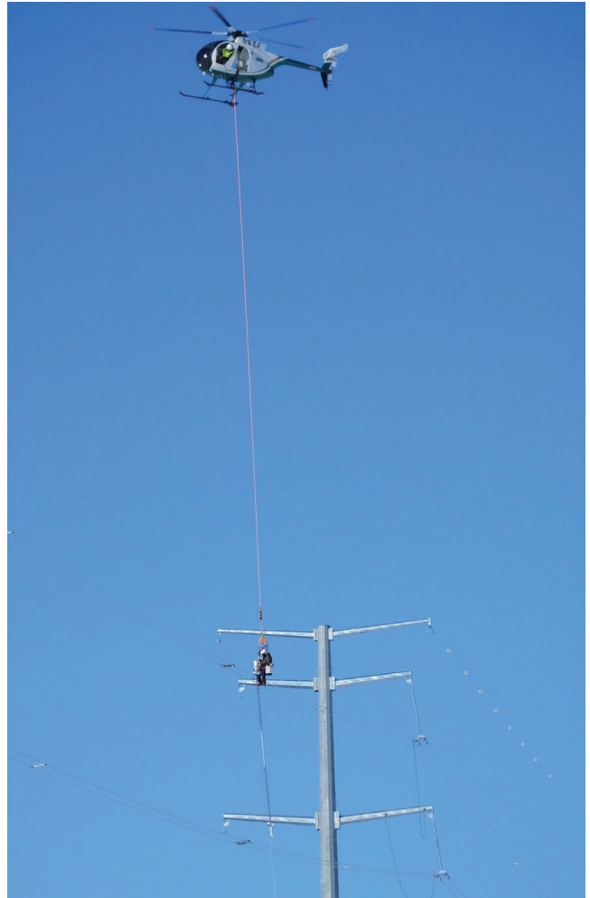
Helicopters may be used to install interphase spacers to minimize ground impact.
