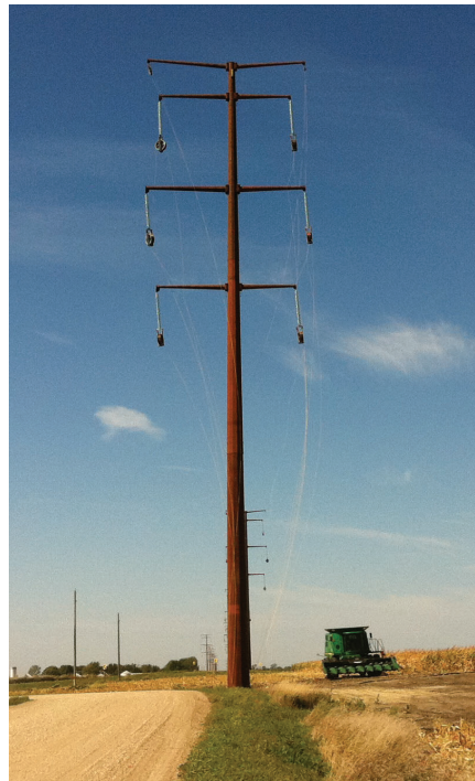
Single pole steel structures were used to reduce land impacts; some locations required two pole structures. Poles are between 140 and 170 feet tall and about 1,000 feet apart. Typically, a 150-foot wide right-of-way was required.
