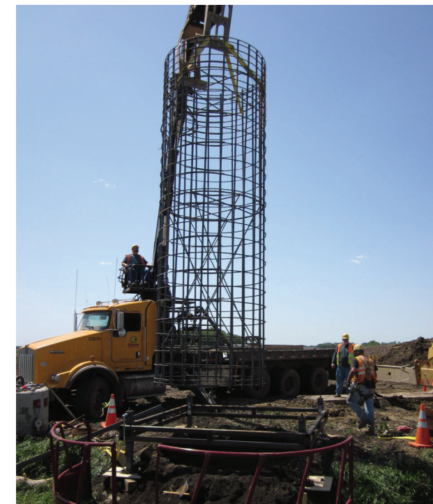
CapX2020 crews install a rebar cage, part of the foundation for steel structures on the Brookings County-Hampton project.
