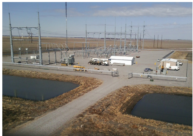
Two new substations were built for the project in St. Cloud, Minnesota and Mapleton, North Dakota. Terminals were added at two other substations.
