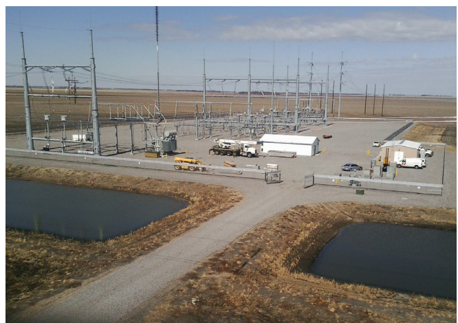
Two new substations were built for the project in St. Cloud, Minnesota and Mapleton, North Dakota. Terminals were added at two other substations.
